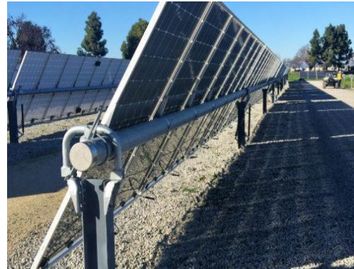
Fig. 6. Single-Axis Tracking Structures. Resource: [Created by the author]
